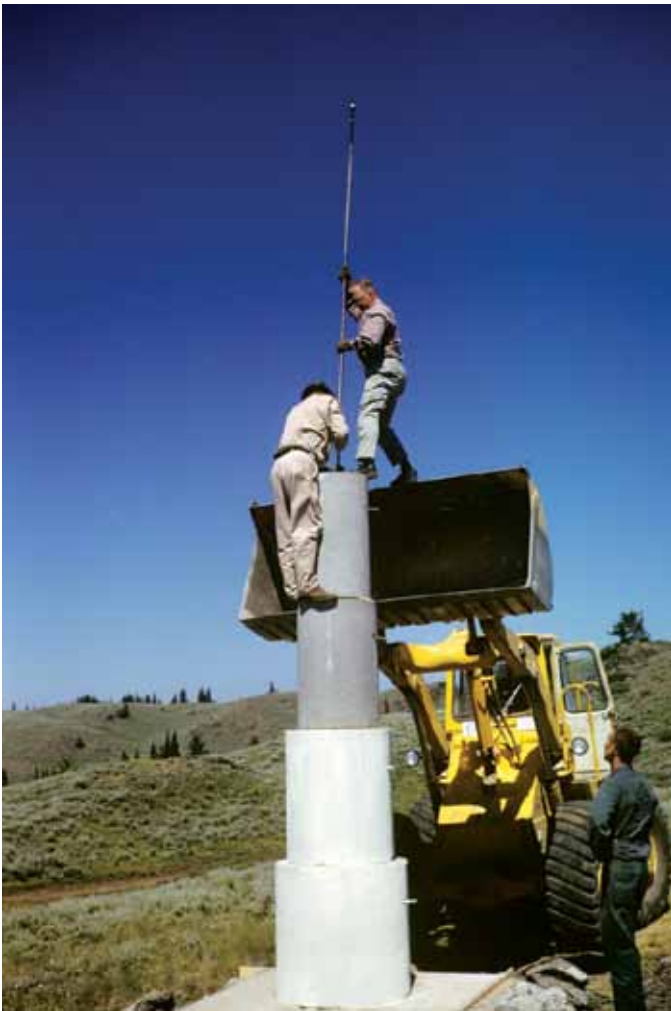
Figure 14 —Snagging the hook seen in Figure 13 with a ring-ended rod that will be used to compress the four concrete cylinders into a rigid pillar to support a solar refractor.
