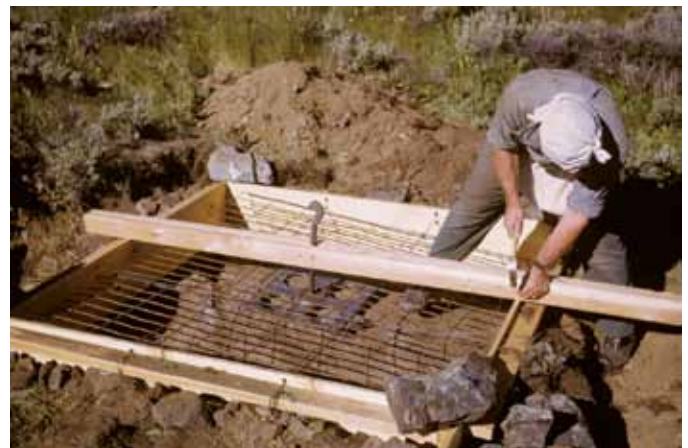
Figure 13 — Mel Lytle builds a form for a cement pad to support a 4-m high concrete pillar for a solar refractor, 1966 July 29.
