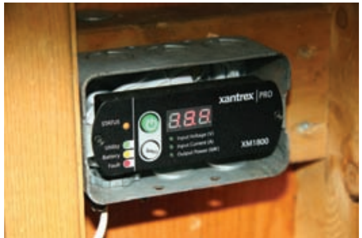
Figure 3 — The remote switch is located beside the door. The readout can show input voltage or current drawn from the batteries.
