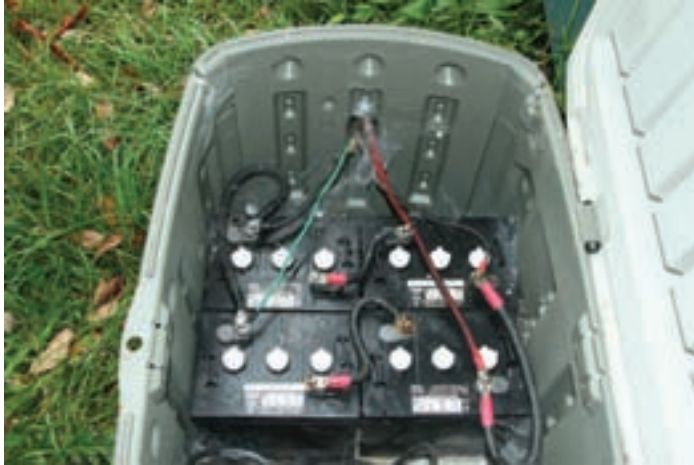
Figure 4 — The batteries live in a Rubbermaid-type garden storage box with vents cut in the ends. Lots of other things live there too. Vents are needed because lead-acid batteries produce hydrogen that is extremely corrosive and even more explosive.
