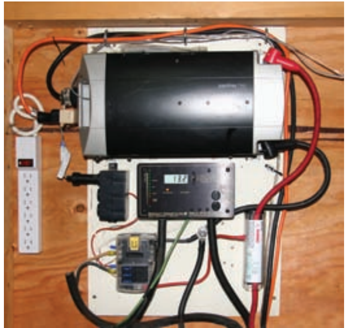
Figure 2 — The inverter and controller mounted on plywood. The plastic cover on the right covers a large in-line fuse for the inverter, and the unit on the left is a multiple fuse block to protect 12-volt circuits.
