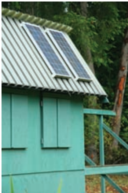
Figure 1 — The roof was built to accommodate the panels. They would need a support frame to get the right angle anywhere else.
