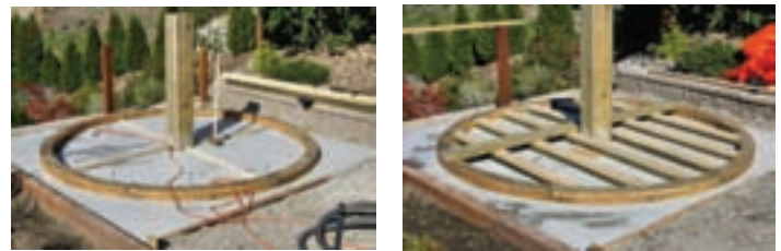
Figure 8 (left) — Base ring and pier installed Figure 9 (right) — Starting the installation of the floor.
