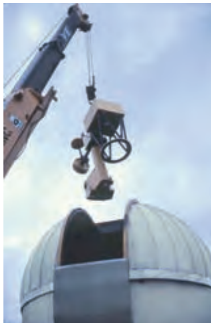
Figure 3 — Loading the dome: the new telescope frame is lowered into place in the Tabor Mountain observatory.
