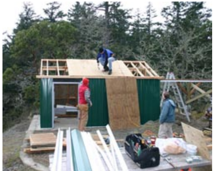
Victoria Centre's Observatory under construction. Roof sheathing starts - Nelson Walker, Charles Banville and Malcolm Scrimger
