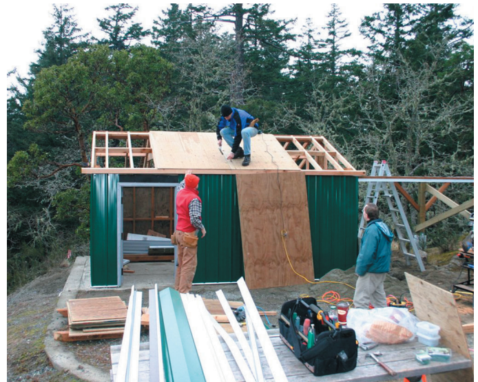
Victoria Centre's Observatory under construction. Roof sheeting starts - Nelson Walker, Charles Banville and Malcolm Scrimger
